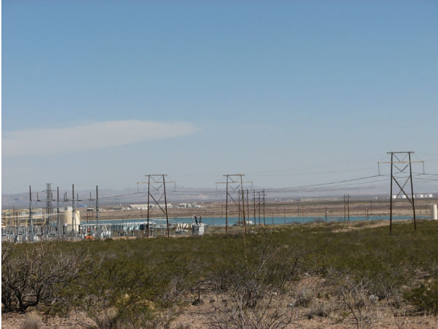
Cooling Tower Reject Water stored in a pond at El Paso Electric Newman power plant in northeast El Paso, TX.
